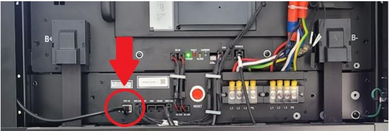
Exposed rear panel of a Samsung Lithium system
